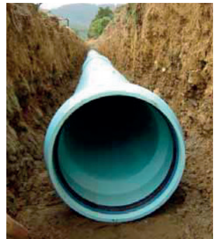
Iplex BLUE RHINO™ in trench ready for backfilling, under sealed road near Levin.
